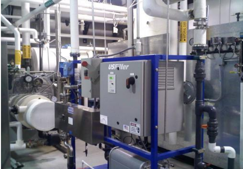
WFI High Capacity Water System and Clean Steam Generator
