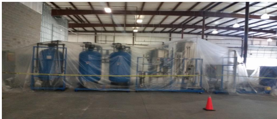
Water for Injection Equipment
