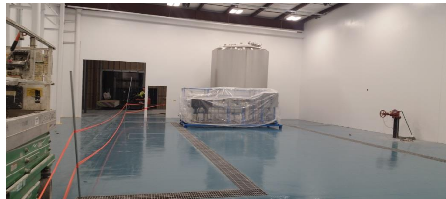
Water for Injection Room
